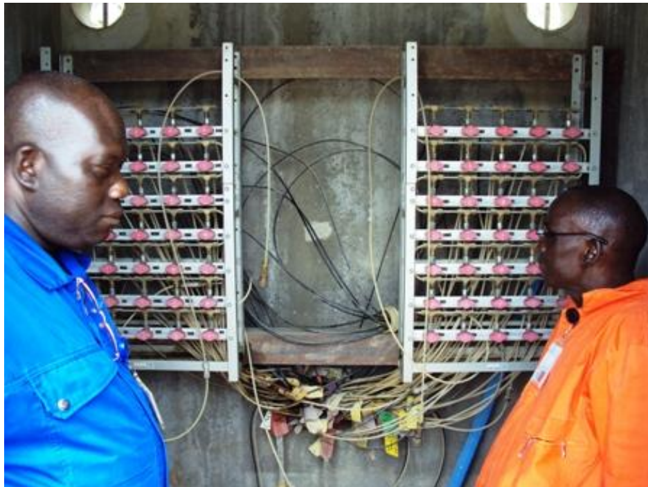
Photo 9.3: Remote-controlled Piezometers Terminals
