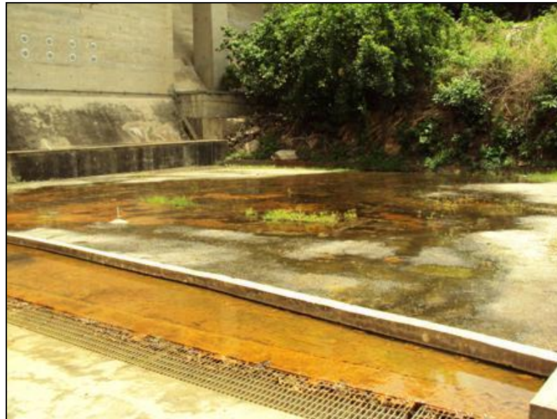
Photo 9.5: Level Area Downstream of Drain AD53 with Spring
