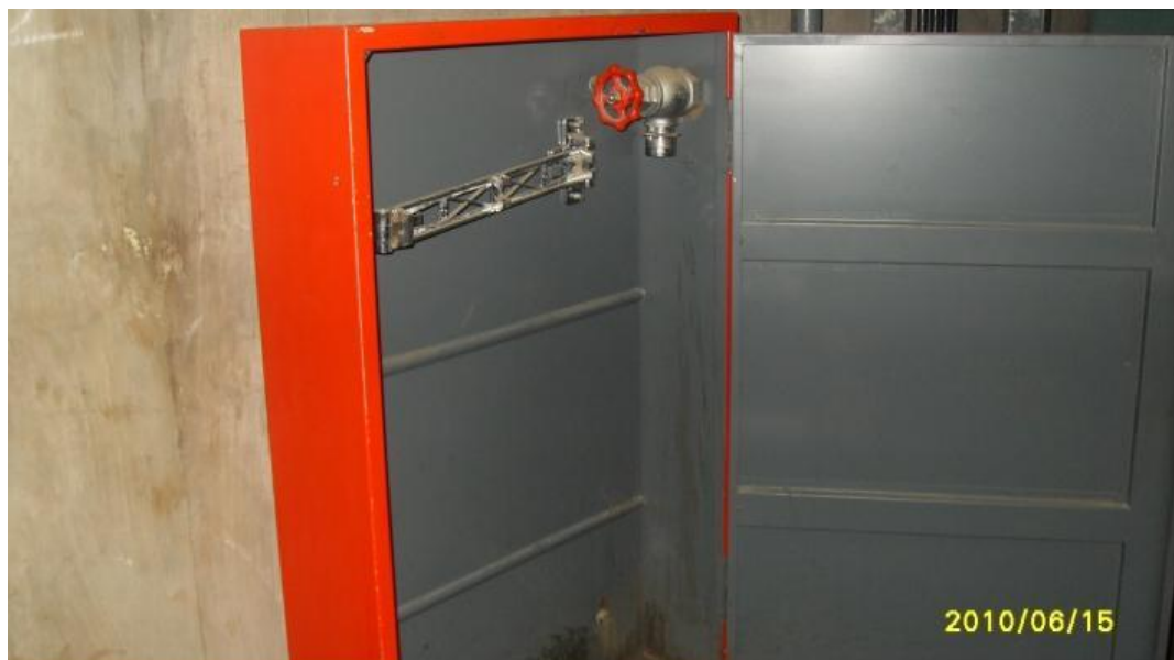
Photo 7.2: Hose Reel Box Without Hose Reel
