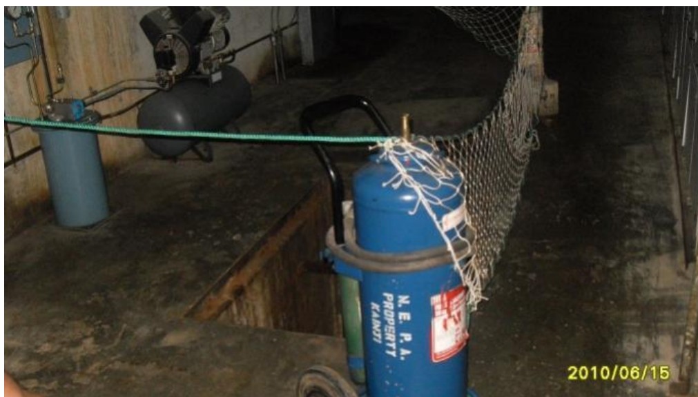
Photo 7.7: Rudimentary Steps to Cordon off Uncovered Chutes
