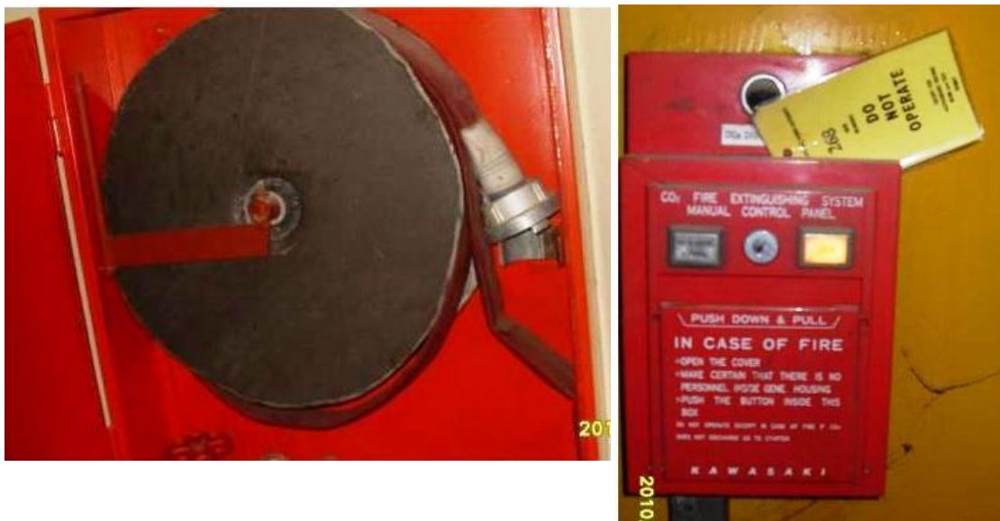
Photo 12.2: Fire Tender Equipment
