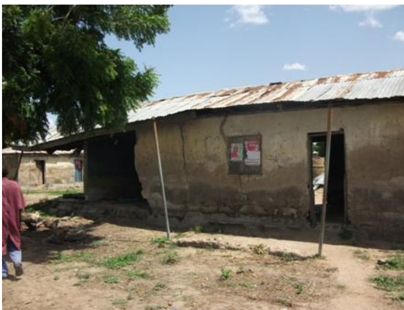
Photo 8.3: Dilapidated House at Awuru Village
