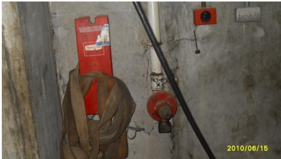
Photo 7.3: Poorly Kept Fire Fighting System
