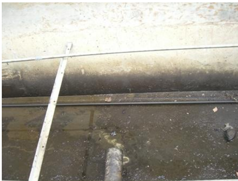
Photo 11.4: Oil Spills into Apron Which Drains to Gutter
