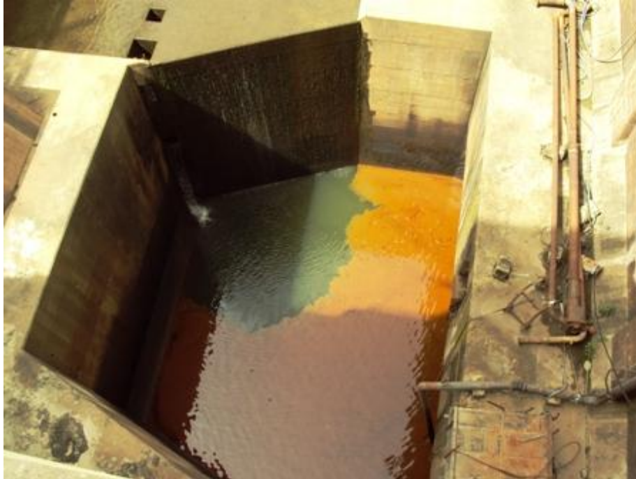
Photo 5.1: Oil Spill in the Open Well of Turbine 4
