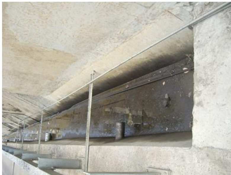
Photo 11.3: Oil Spills into Gutter Which Drains to River Niger
